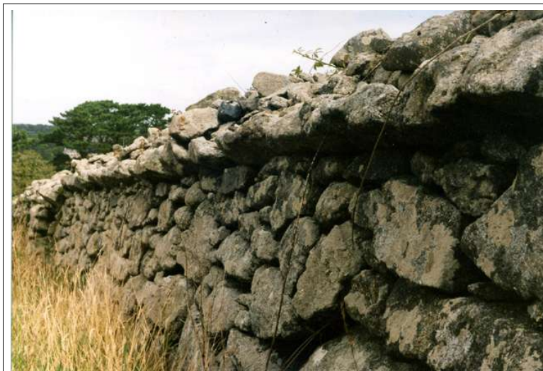
Stone hedge built with a coping on the park side to deter deer from jumping out.
