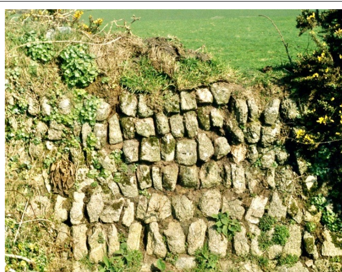
A good farmer-repaired gap (centre, upper four courses) using the original stone which had fallen from the hedge.. Note style of repair matches original, Grassy tobs placed on top.
