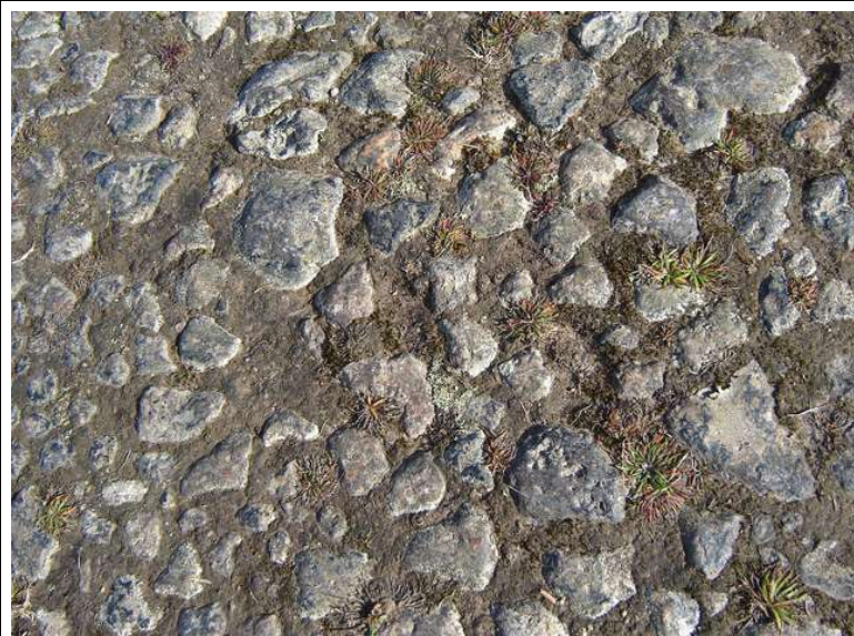
A close view of the pre-tarmac rolled stone surface of the old St Just coach-road, still sound and good today.
