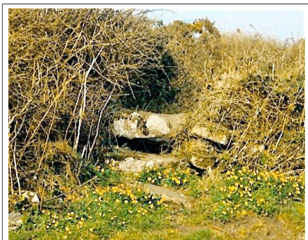
This shows what can happen if foot-stones are not firmly bedded in. The foot-stone shown here has sunk at the right-hand side and needs to be levelled up as it makes the stile very awkward to use especially when wet and slippery. Good building saves remedial work later.
