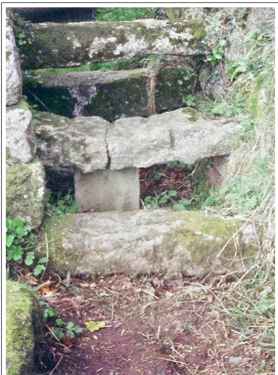
Safe support of cracked tread with a reinforced concrete block saves expense of replacing tread, retains original stone and avoids unsuitable replacement with wooden stile.
