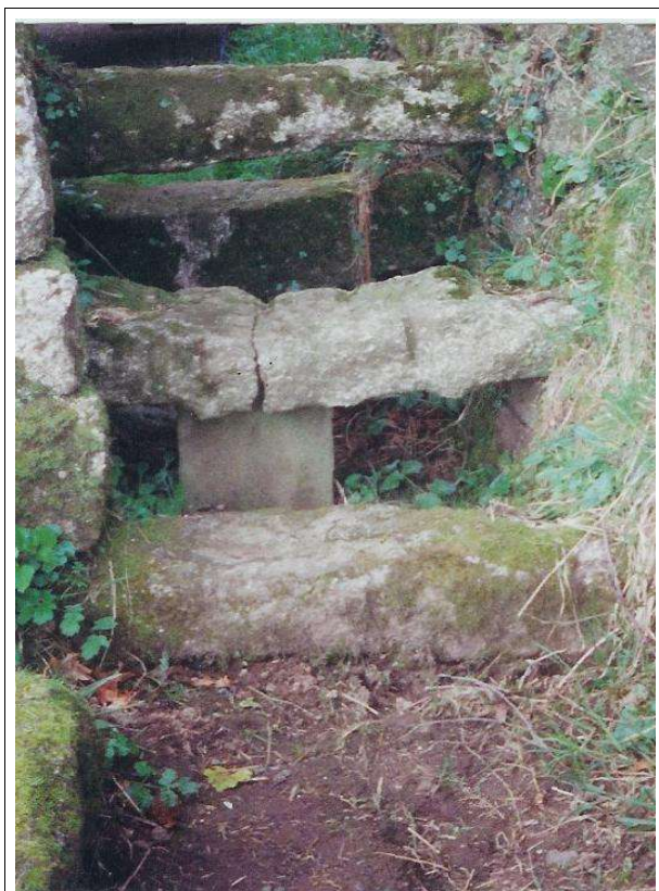
Safe support of cracked tread saves expense of replacing tread, retains original stone and avoids unsuitable replacement with wooden stile.
