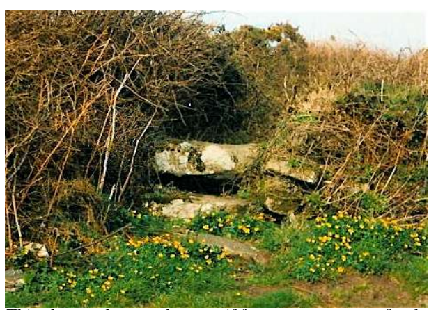
This shows what can happen if foot-stones are not firmly bedded in. The foot-stone shown here has sunk at the right-hand side and needs to be levelled up. Good building saves remedial work later.
